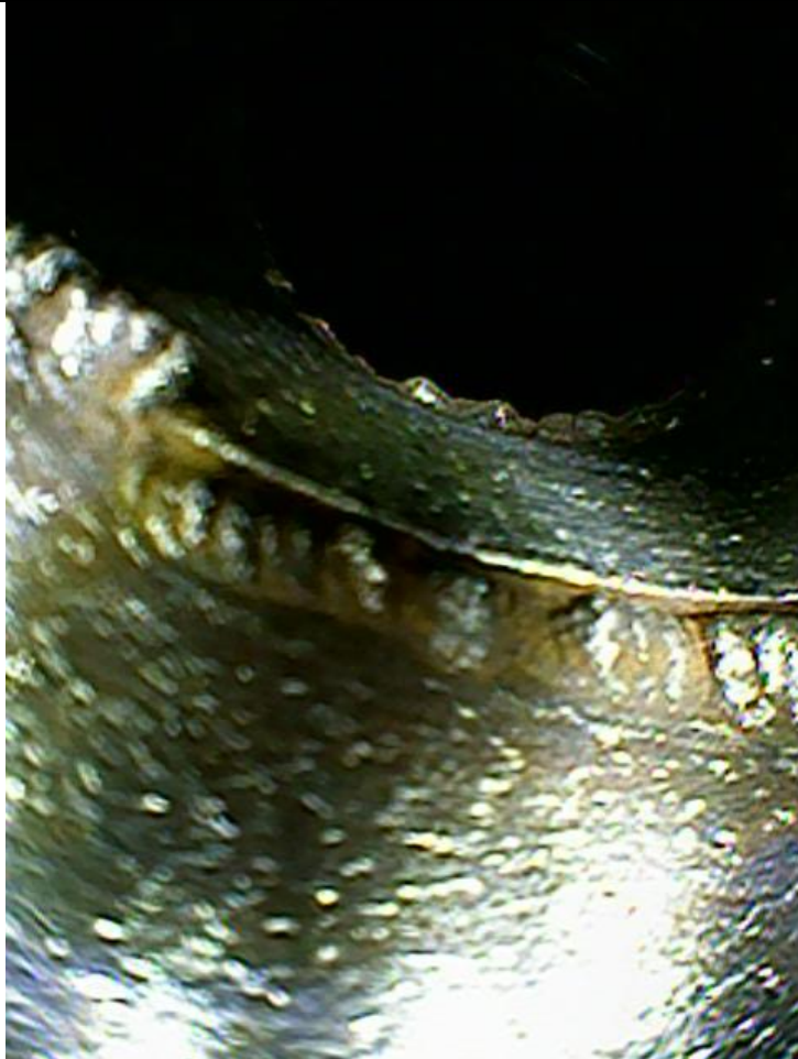
Potential point of leakage at butt joint
