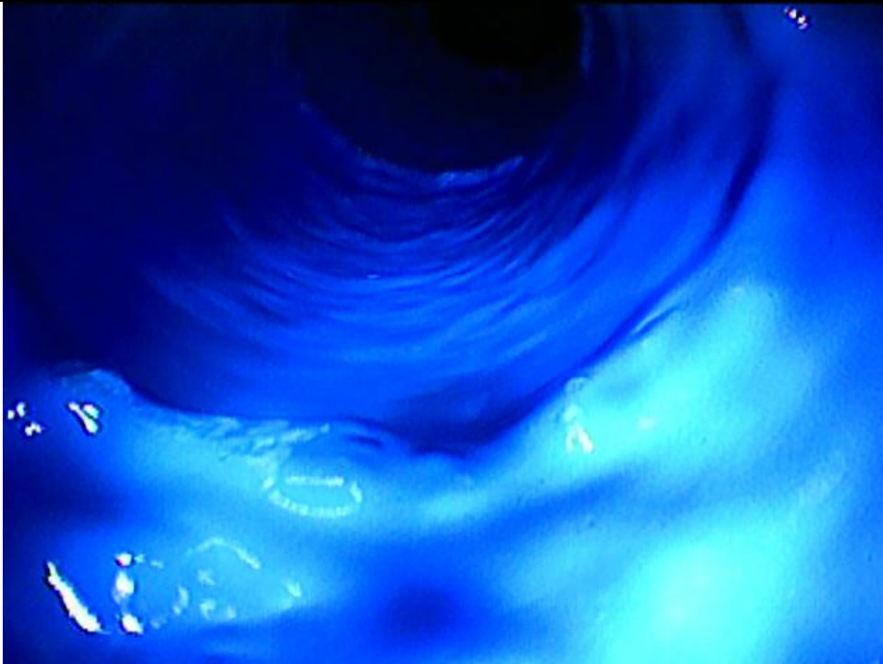
Welded joint showing good monolithic coverage
